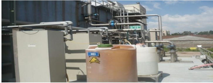
Figure 27 BGI waste water treatment site
